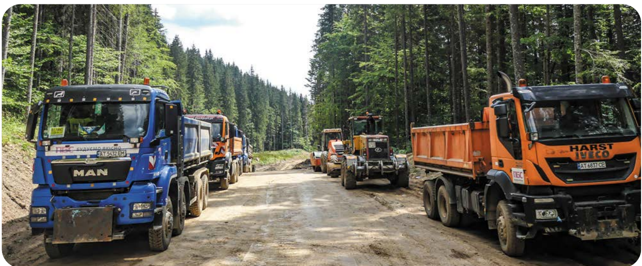
New “forest highway” under construction on 22.08.2023, two weeks before the contract with PBS was signed
